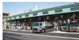
Shikoku Operations Lorry loading facilities
